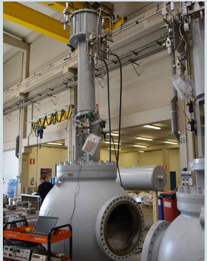
Fig. 9: 28" hot gas bypass valve and anti-surge for petrochemicals Emergency time <2 seconds. Control time <5 seconds without any overshoot
