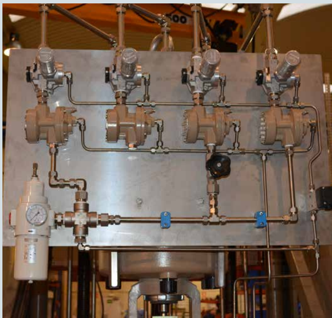
Fig. 1: Example of an anti-surge control panel
